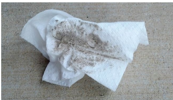
Dirt on Sub Floor
